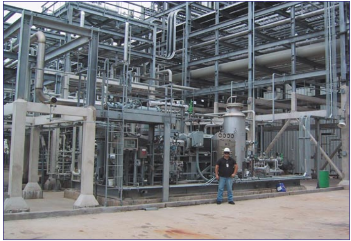
Figure 4. Isobutane nitrogen recovery unit.
