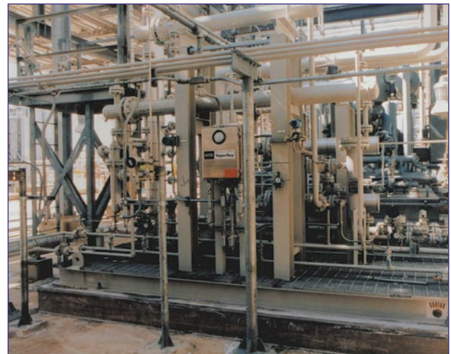
Figure 6. A hydrocarbon recovery unit.
