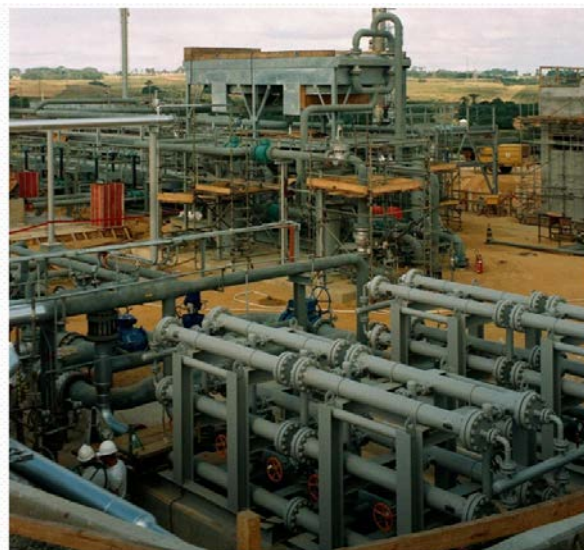
Figure 6. Photograph of the Membrane system at El Paso combined cycle utility power plant.
