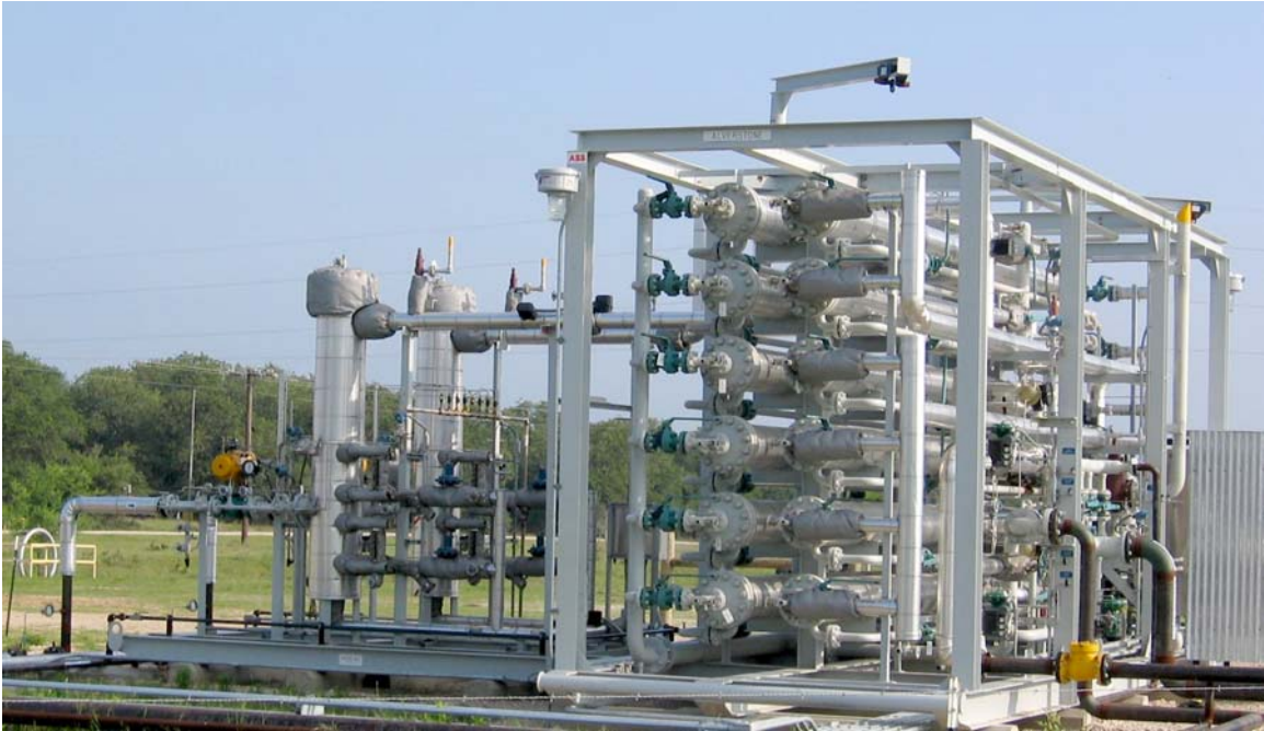
Figure 4. A standard CO 2 treatment skid with pretreatment filter/separators on adjacent skid to left.
