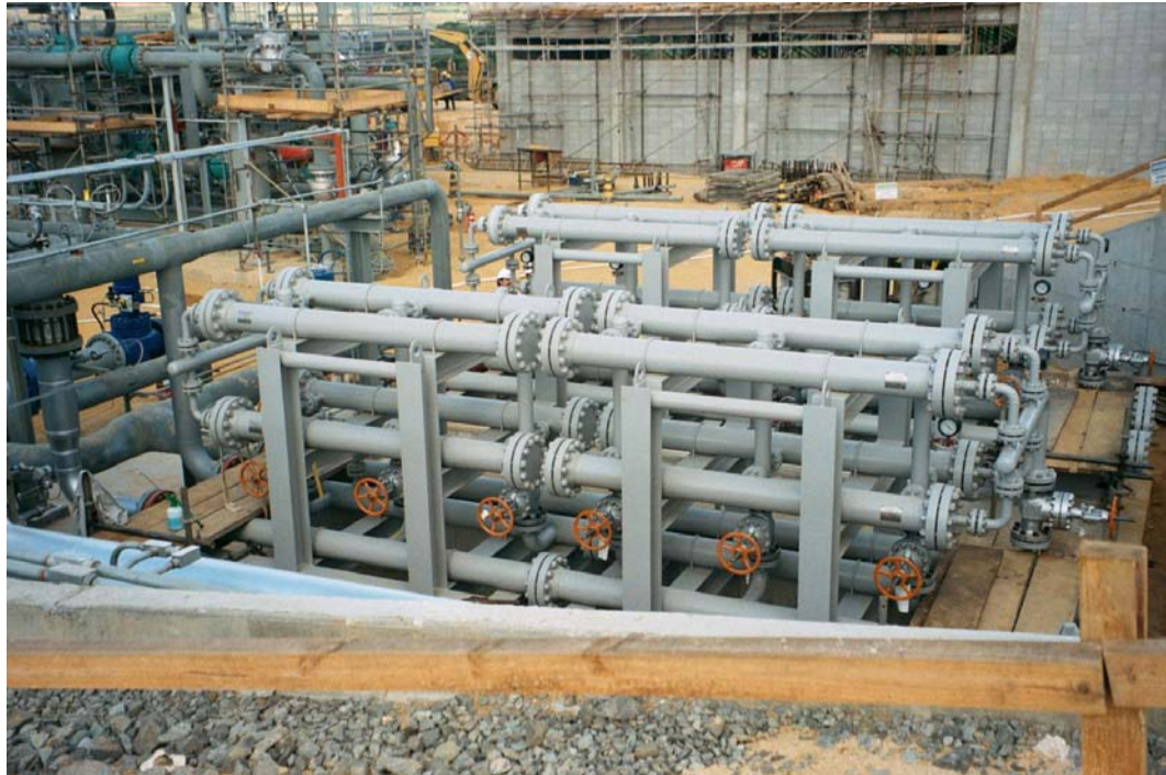
Figure 3. A typical membrane skid; sixteen carbon steel pressure tubes house the membrane modules.
