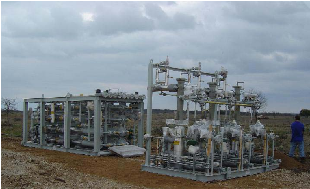
Figure 8. Photograph of the first full-scale commercial system under installation for North Texas Exploration in 2004.
