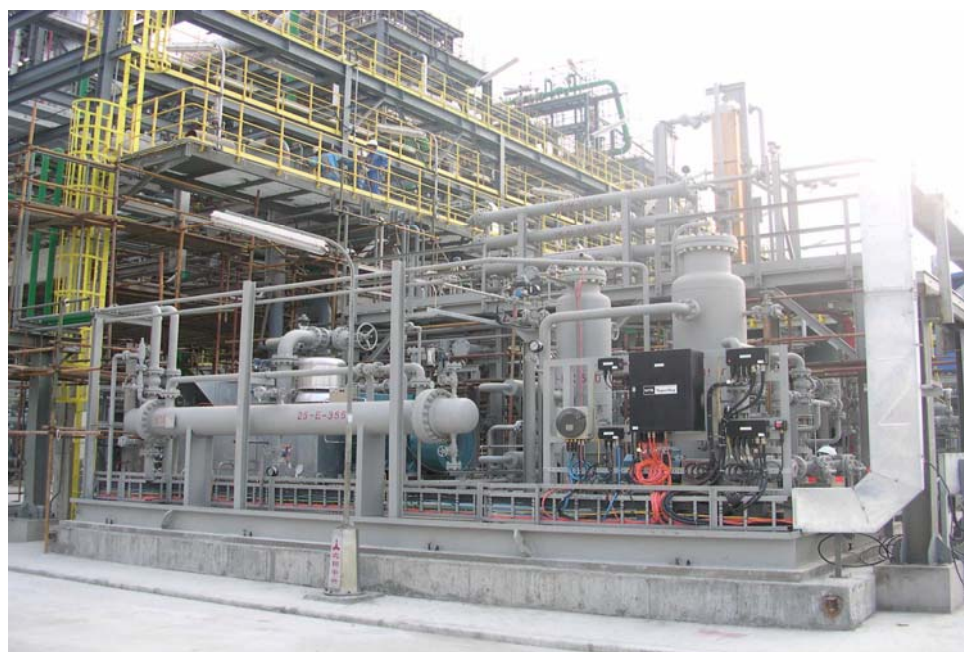
Figure 7. Photograph and process flow diagram of a membrane propylene recovery system installed at a modern polypropylene plant. The front portion of the unit is the compressor package. The spiral-wound membrane modules are contained in the horizontal tubes above and behind the compressor. This unit recovers approximately 1,000 lb/h of hydrocarbons.
