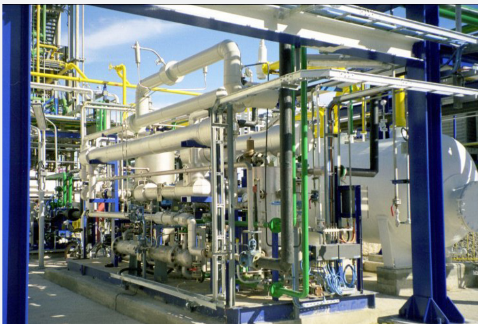
This VaporSep® system recovers 1000 tons per year of VCM.
