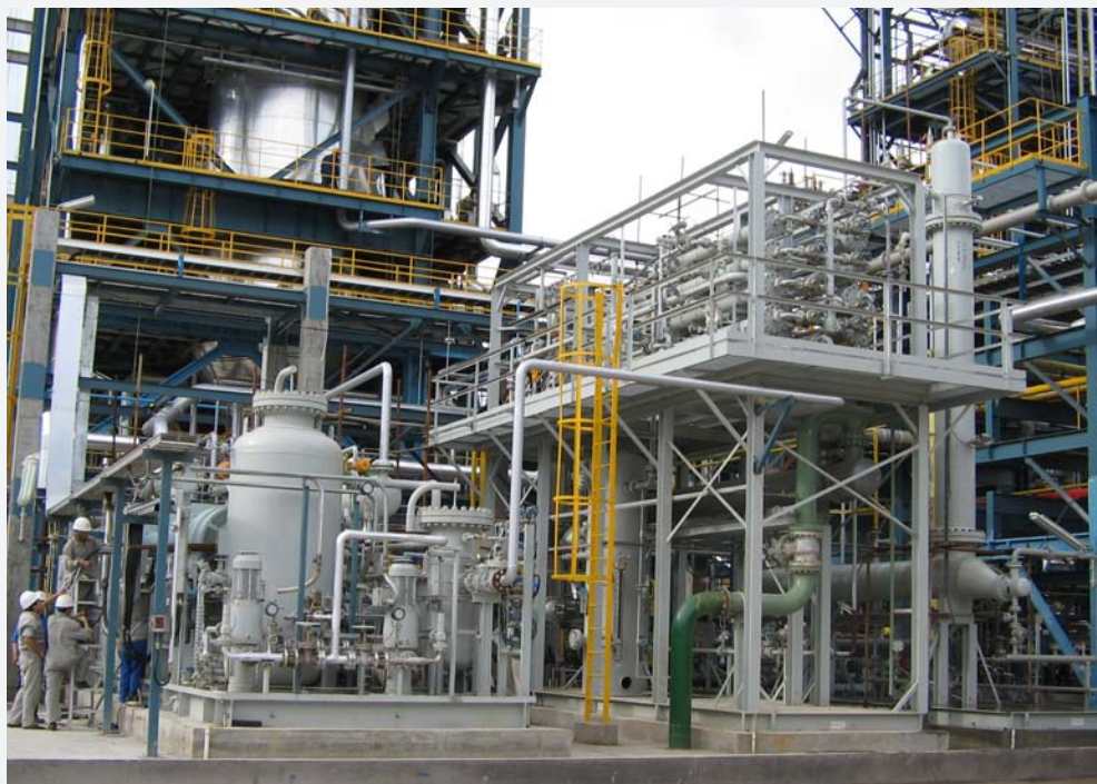
This unit recovers isobutane and nitrogen in a modern polyethylene plant
