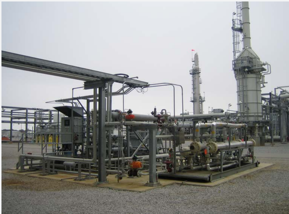
Demonstration LPG-Sep™ unit operating at a US Gulf Coast location
